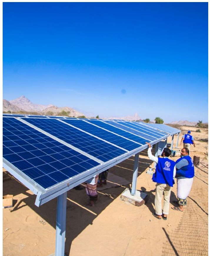
IOM WASH engineers inspect newly installed solar panels in Abyan ©IOM 2020 / R. Ibrahim
