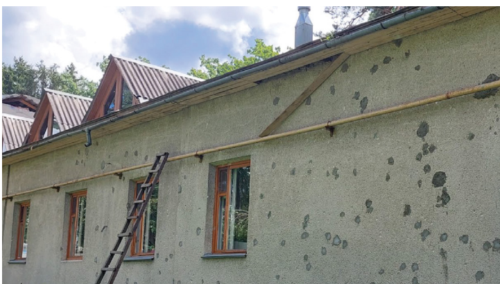
In preparation for the cold season, IOM carried out repairs in a former summer camp in Irpin, heavily affected by the war. The camp currently serves as a collective centre
