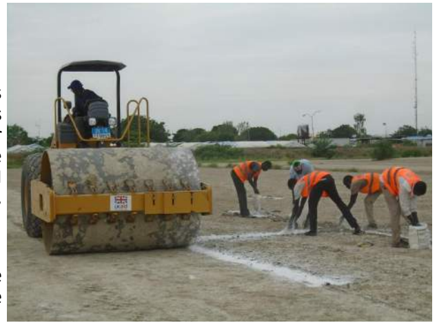
IOM CCCM staff recently took the lead to develop a temporary helicopter landing site in Malakal to ensure that humanitarian staff and supplies could safely arrive in Malakal.
