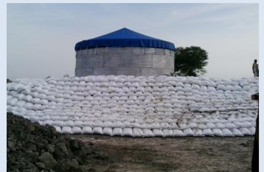
IOM completed preparation of a T70 water tank in Sector 3 of the extension site.
