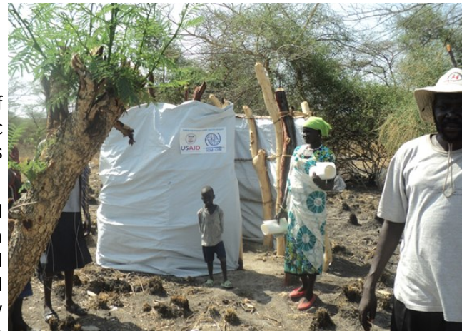
IDP women appreciate the privacy provided by the emergency showers built by CMD.
