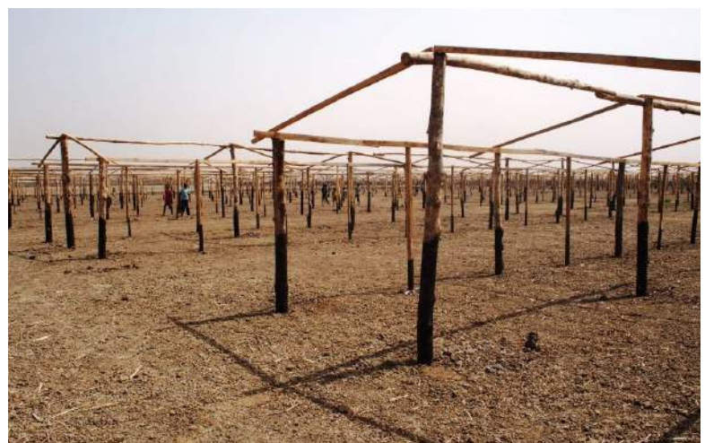
IOM partner Concern erected shelter frames at the Bentiu PoC expansion site, using shelter material from the IOM pipeline.
