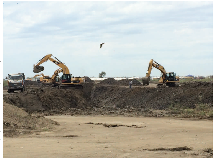
IOM constructs retention basin to prevent flooding at Bentiu PoC expansion site during the rainy season
