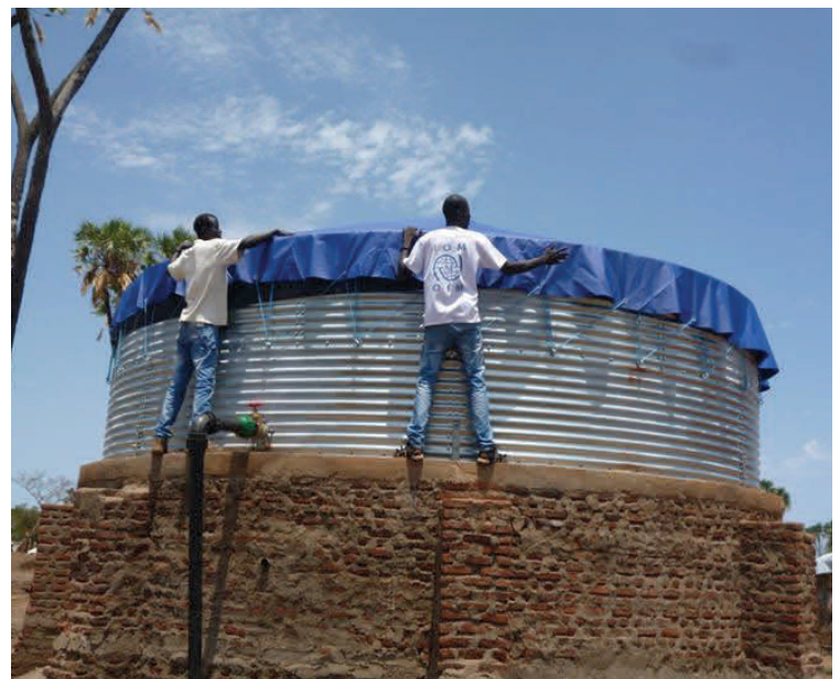
Water reservoir tanks at Doro refugee camp.
