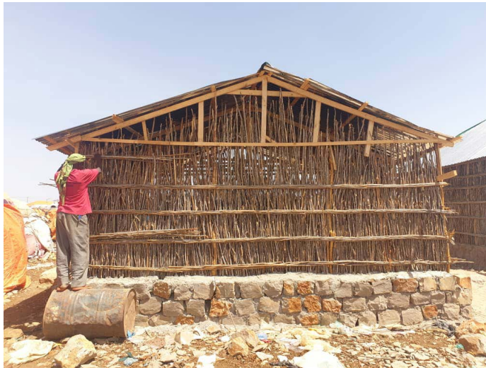
A beneficiary trained in shelter construction building a robust shelter in Baidoa.
