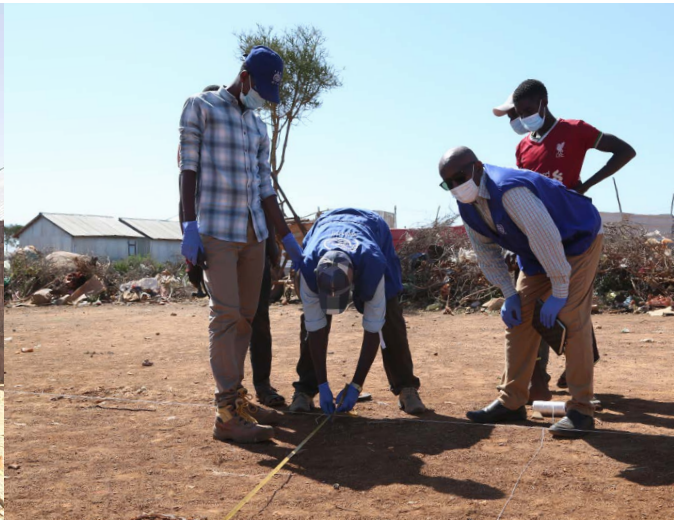
IOM staff begin demarcations of plots to build robust shelters in Baidoa.
