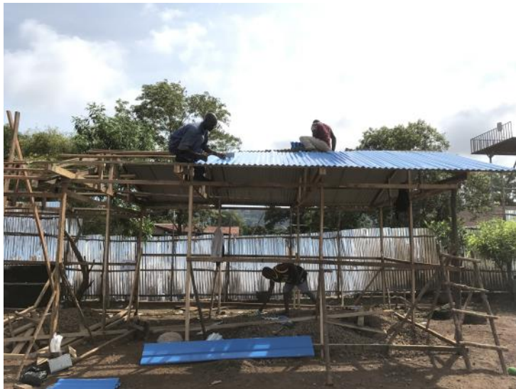
A shaded area being constructed at Juba transit site IOM 2017 (Photo: Haruka Ueda)
