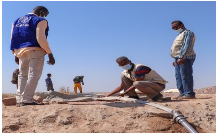
IOM staff test the water supply points in Um Rakuba Camp, Sudan © IOM 2020
