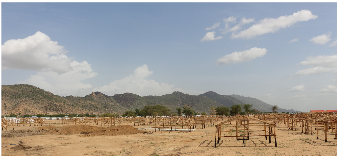
Since 2016, IOM has constructed more than 3000 shelters to support displaced populations in Pulka, North-East Nigeria. To better assist displaced populations in transit and reception sites, IOM is currently constructing an additional 700 shelters in Camp C. (IOM/2018)
