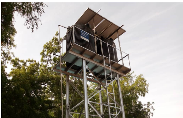
Solar-powered borehole in Gwoza © IOM 2019
