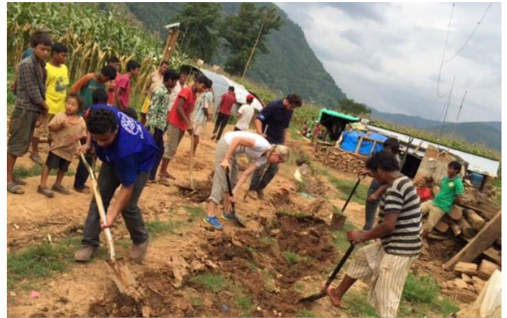
The site planning team at work with local volunteers in Bhimtar (© IOM 2015)
