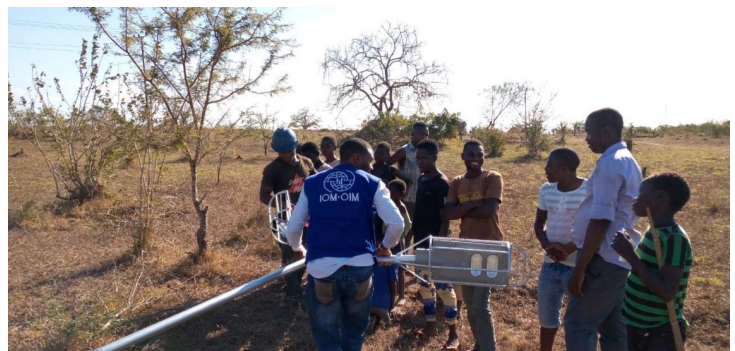
IOM Protection and CCCM team installs solar lamps in Tratara, and Chuiba sites. © IOM 2019
