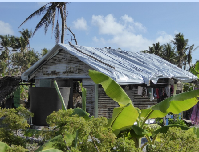
USAID plastic sheeting is used to cover a family home in Faderai, Yap, FSM © IOM Micronesia 2015
