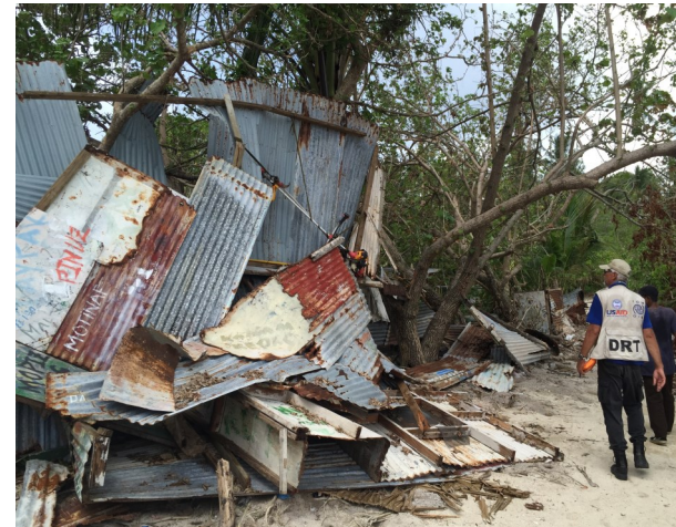
IOM Disaster Response Team assesses damage in Chuuk, FSM © John Schroer 2015
