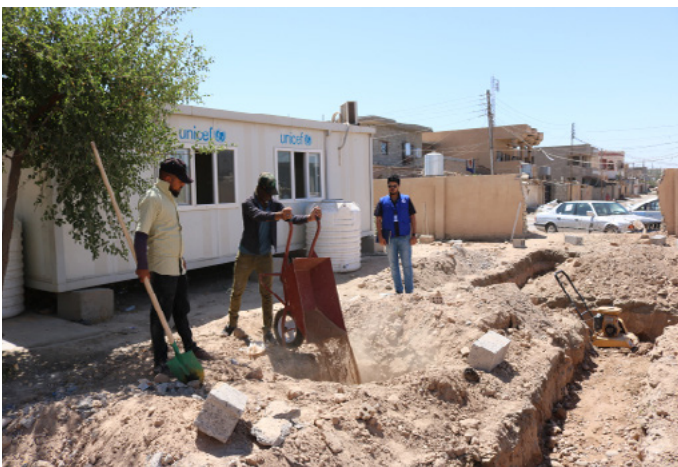
IOM staff following up during the first stages of building three additional classrooms for Al Ahrar Primary School in Al Firdous Community, which is the only school in the neighborhood.
