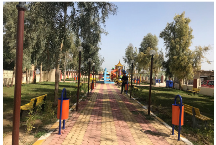
IOM rehabilitated the park in Gwer sub-district, including rehabilitation of electricity and water networks, and providing and installing other necessary equipment.
