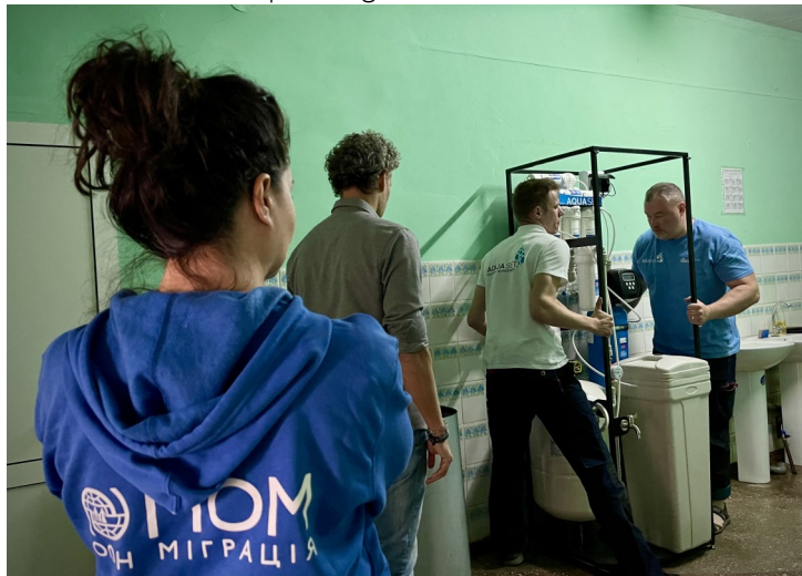
IOM Ukraine and its implementing partner install a water treatment unit in a collective centre in Vinnytsia. © IOM 2022
