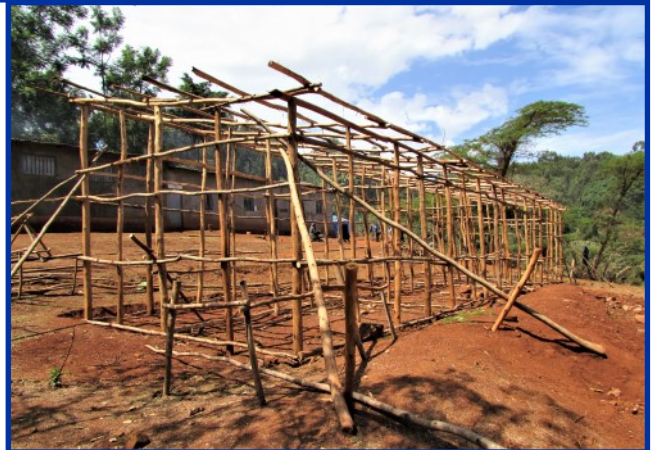
A COMMUNAL KITCHEN UNDER CONSTRUCTION IN WESTERN STAR SITE, WEST WOLLEGA © IOM 2019/Z.HDIDOU
