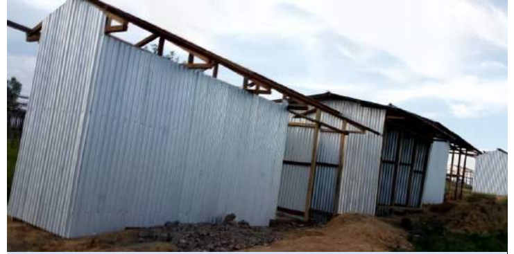
Construction of reinforced emergency latrines in the Lycee Kigonze site in Bunia, Ituri province. © IOM 2019
