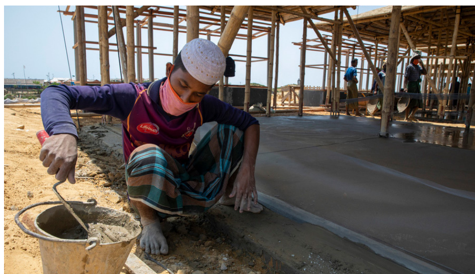
IOM volunteers work to construct COVID-19 Isolation and Treatment Centers in Cox's Bazar, Bangladesh. © IOM 2020
