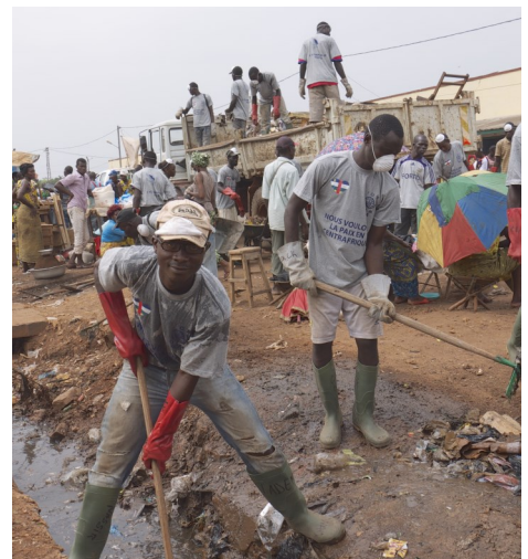
IOM launched a cash-for-work street cleaning project in Bangui. © IOM 2014 (Photo: IOM CAR)
