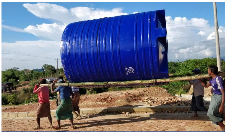
Transporting the water tank to construct the small-scale water network at Camp 20 Extension. © IOM 2020
