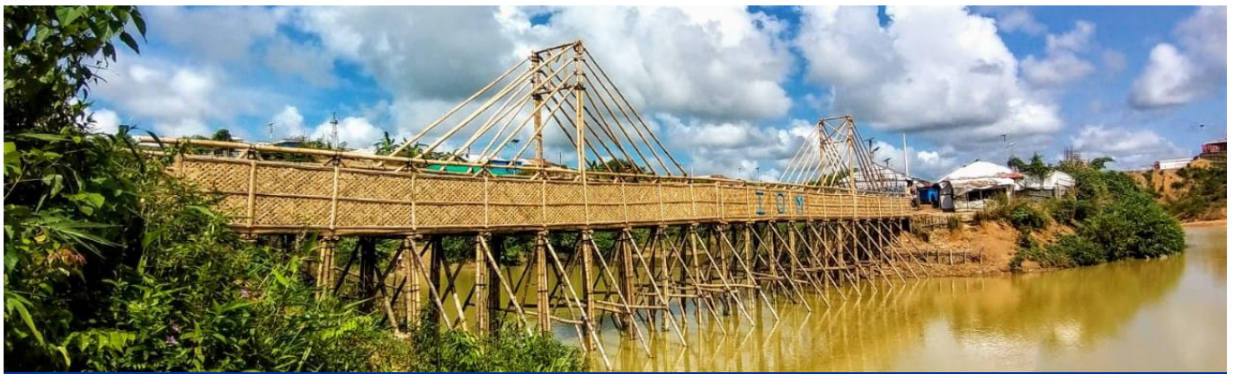
This month, the team repaired the bamboo bridge connecting the hospital from Camp 20 to Camp 18. © IOM 2020
