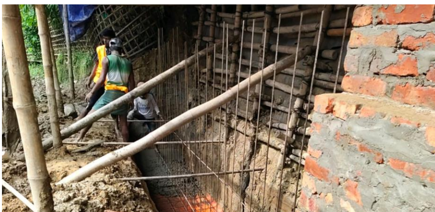
A total 172m 2 of drainage installation has been completed in Camps 22, 24 & Nayapara in Teknaf. © IOM 2020
