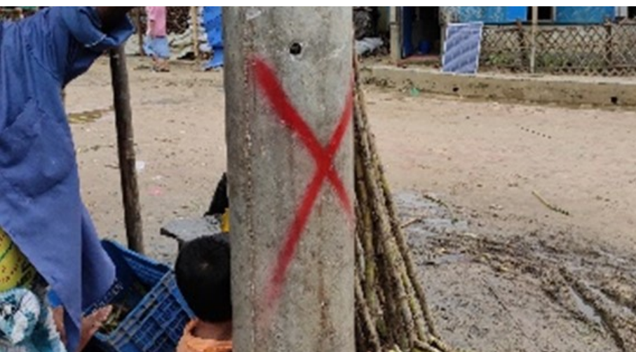
A MINI-GRID NETWORK POLE CROSSED OUT FOR RELOCATION AS IT IS PLACED WITHIN ROAD ALIGNMENT BY NEARBY PAN BAZAR ROAD IN CAMP 9 © IOM 2019
