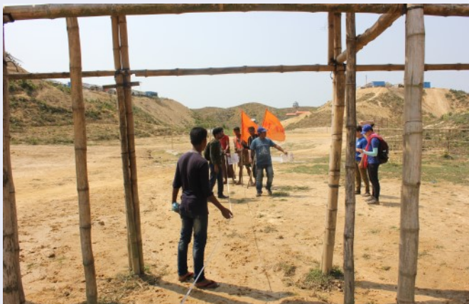
THE SITE PLANNING TEAM DISCUSSES WITH IOM SITE DEVELOPMENT TEAM THE POSITION AND SPECIFICATIONS OF THE MAIN DRAIN. ©IOM 2019/MARIEL KISLIG
