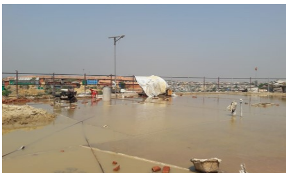
BASE SLAB CASTING COMPLETE AT RESERVOIR SITE FOR WATER PIPELINE NETWORK IN CAMP 12 ©IOM
