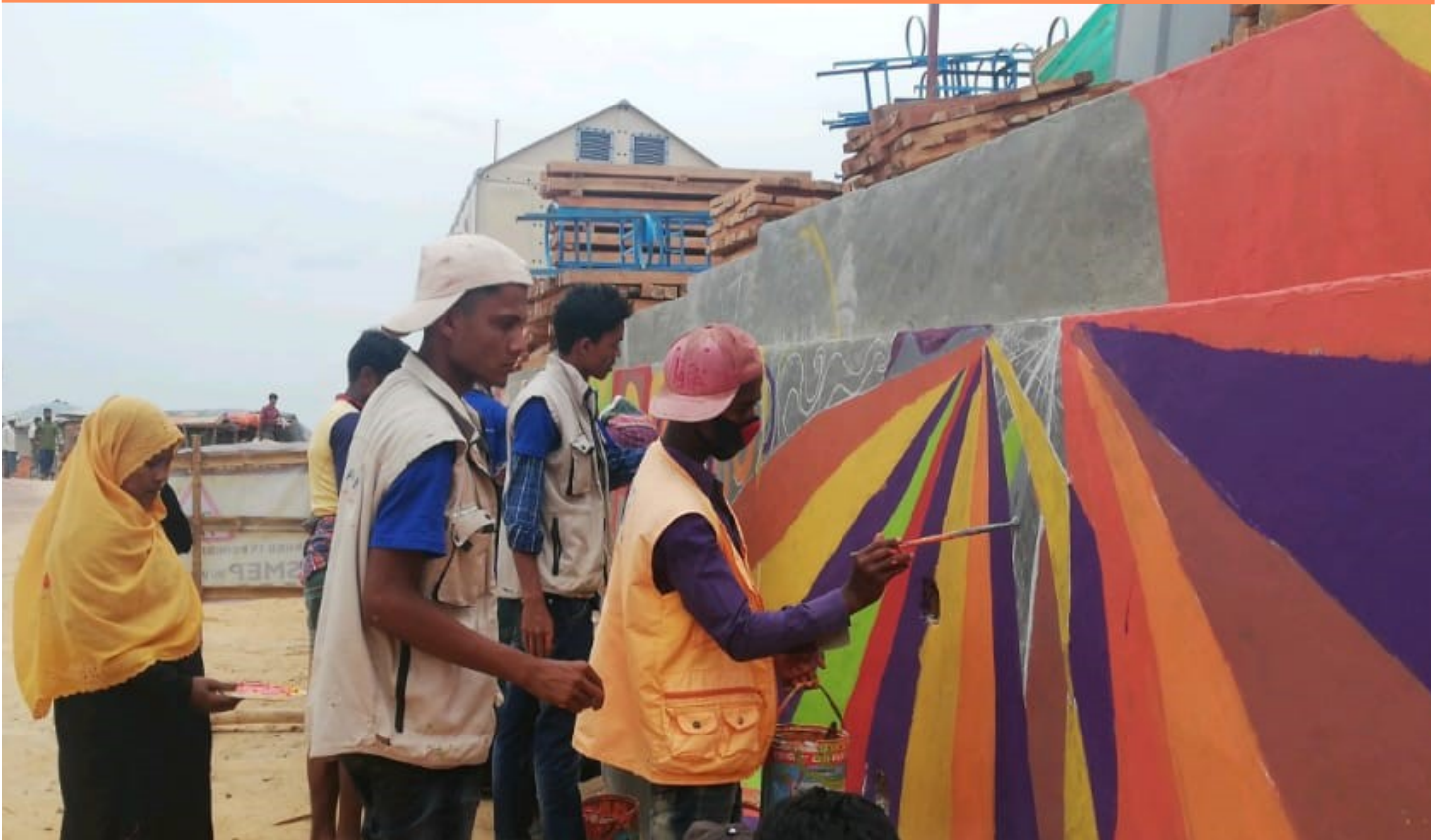
SMEP VOLUNTEERS WORKING WITH IOM MENTAL HEALTH PSYCHOSOCIAL SUPPORT PARTNER, ARTOLUTION, TO PAINT 100M OF RETAINING WALLS ON THE MAIN ROAD ©IOM 2019
