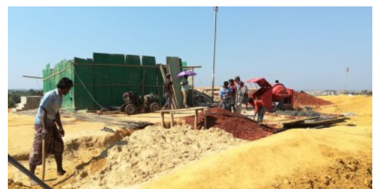
PLATFORM CONSTRUCTION AT THE RESERVOIR SITE FOR THE WATER PIPELINE NETWORK IN CAMP 12. ©IOM 2019
