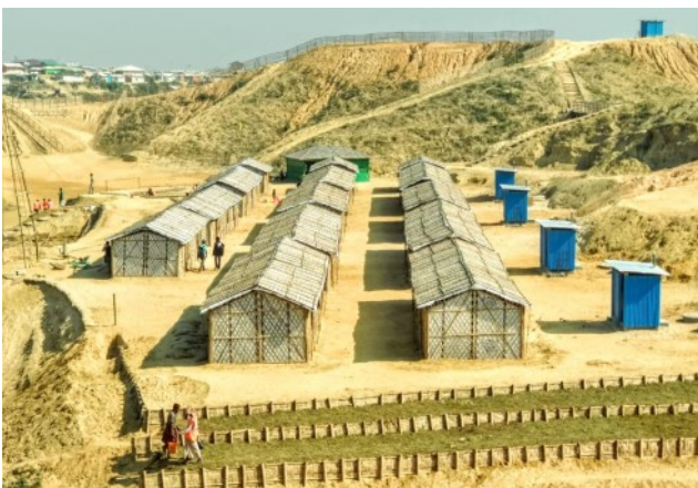
AFTER SHELTER AND WASH FACILITY DEMARCATION, SITE STABILIZATION AND GRASSING WORK IS ONGOING IN CAMP 20 EXTENSION. ©IOM 2019
