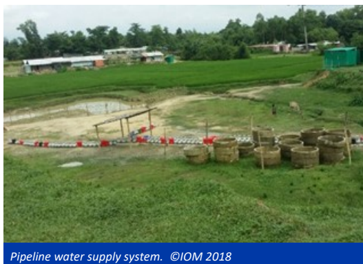
Pipeline water supply system. ©IOM 2018
