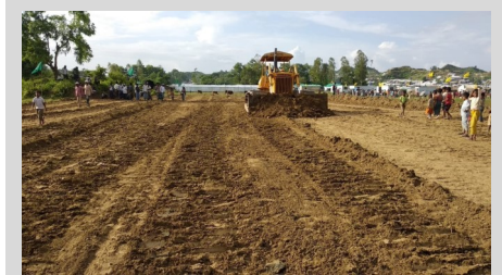
Site Maintenance and Engineering Project (SMEP) preparing site for the relocation of households at risk of landslides.
