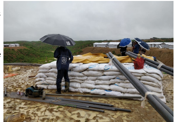
Installation of the second water emergency system in Camp 20 Extension. ©IOM 2018/Rigan Ali Khan
