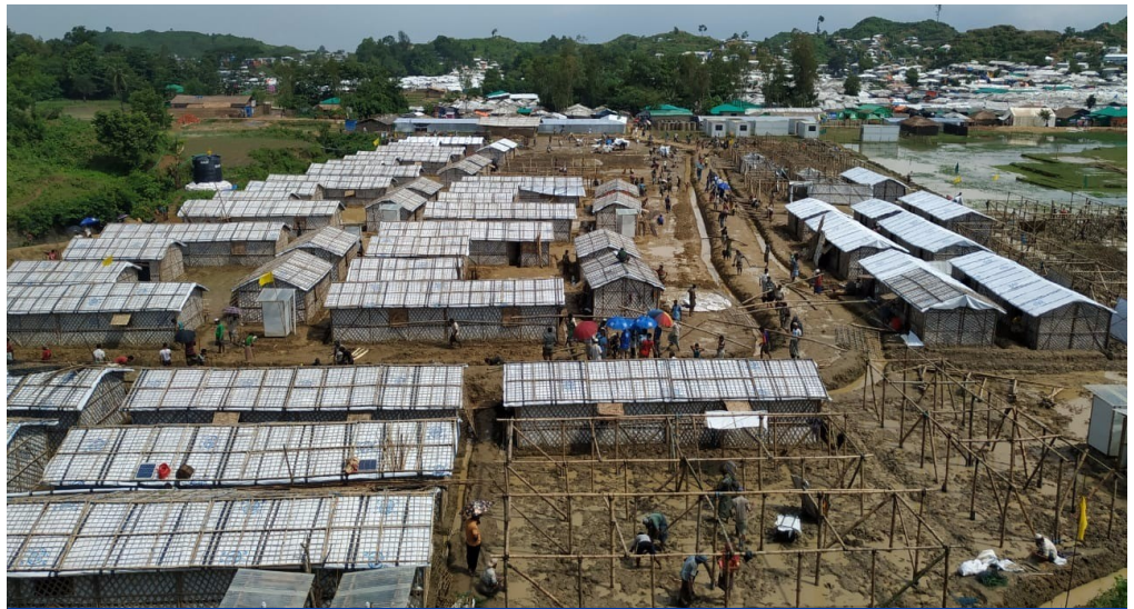
IOM is hiring over 250 Bangladeshi workers per day, and constructing 150 Robust Emergency Shelters to relocate the most at-risk families in Unchiprang ©IOM 2018
