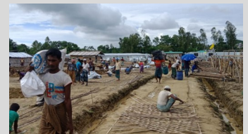
Relocations have started for the families from the most at-risk areas in Unchprang.
