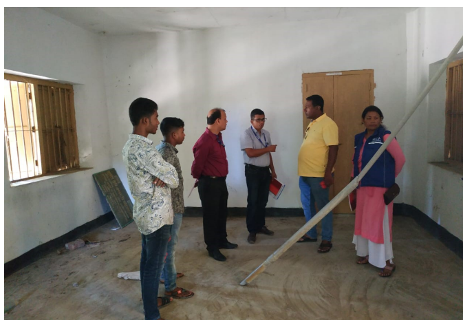
IOM team visiting the renovation activities of Cyclone Shelter in Hariakhali, Subrang Union. ©IOM 2018
