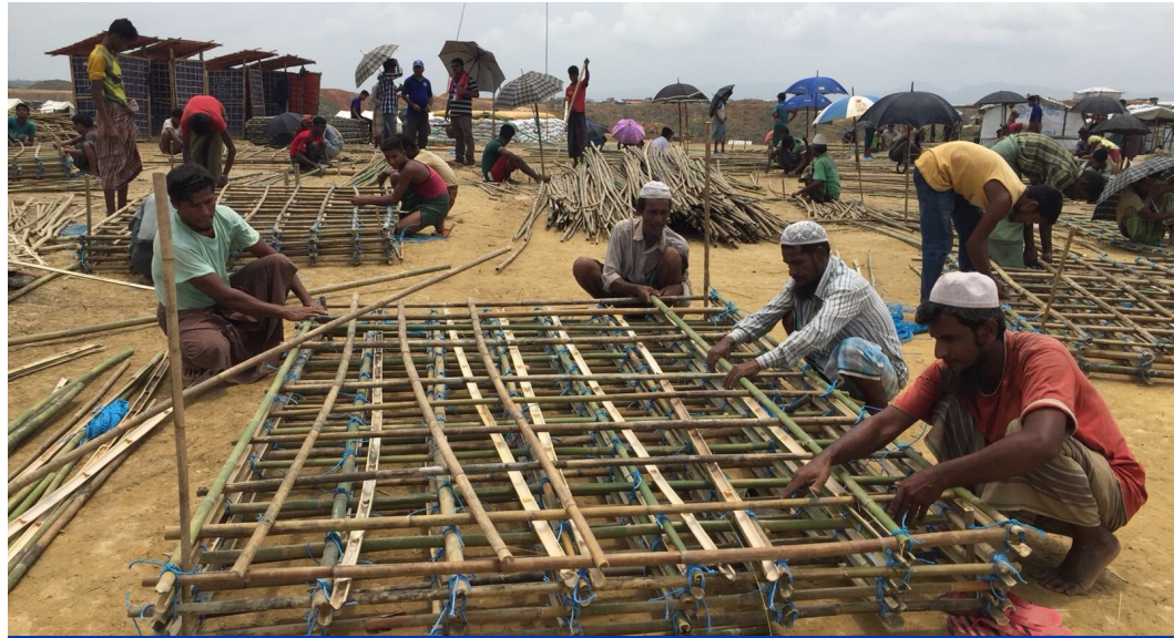
Shelters are being constructed in Camp 20 Extension for households at highest risk of natural hazard and prioritized for relocation. ©IOM 2018/Josh Hart
