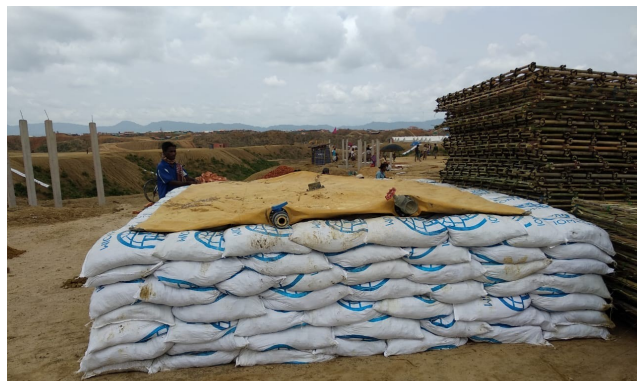
A second bladder tank is being installed in Camp 20 Extension to provide another 5,000 liters of water to beneficiaries every day. ©IOM 2018
