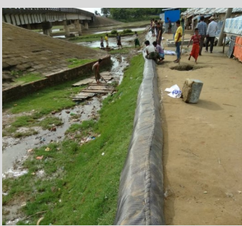
In preparation for the planned high tide, soil was extracted from the river and wrapped in Geotextile to elevate the protection dike in Purbo Assarbonia in Shamlapur.
