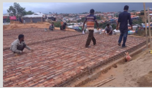
Reinforcement setting in Camp 10 of the floor casting of a health post.
