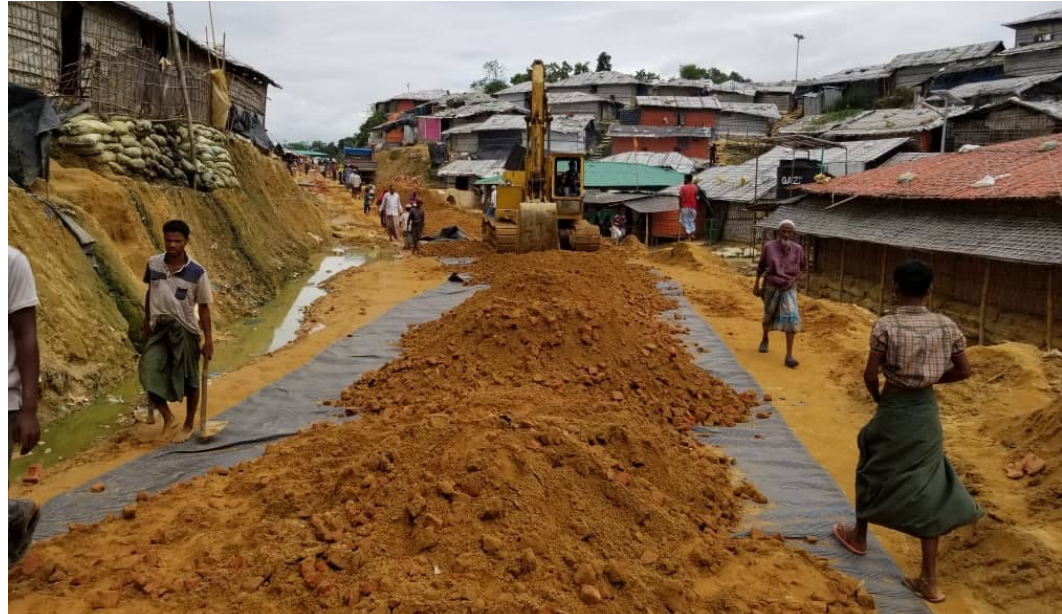
Construction of road #2 in Kutupalong Balukhali Expansion Site by IOM Site Development. ©IOM 2018
