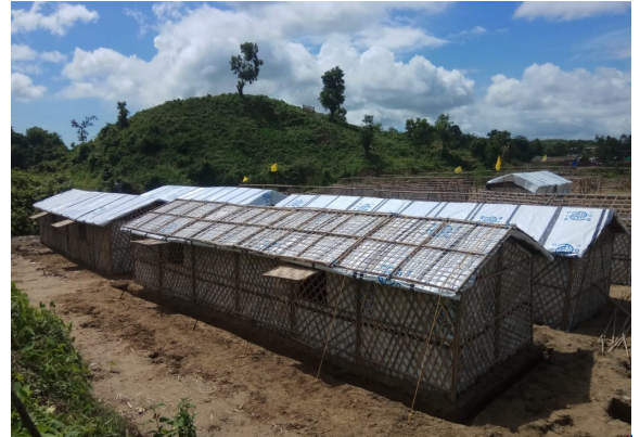
IOM has constructed 1,293 Robust Emergency Shelters in Camp 20 Extension. Another 150 shelters have been started in Unchiprang. ©IOM 2018
