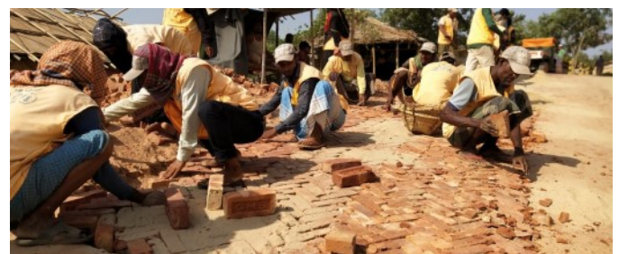
SMEP VOLUNTEERS REPAIRING OLD SECTIONS OF BRICK ROAD IN CAMPS 2 AND 2W ©IOM 2019
