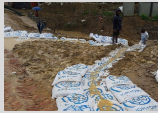
Water diversion channel at UB3 inlet side to protect culvert head wall from seepage and soil erosion.
