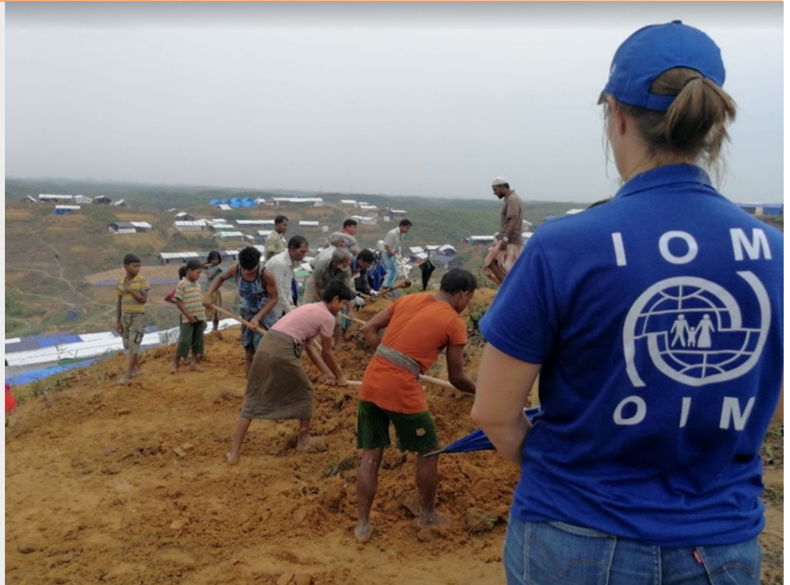
IOM Site Development is working to improve road access across the displacement sites. @IOM 2017
