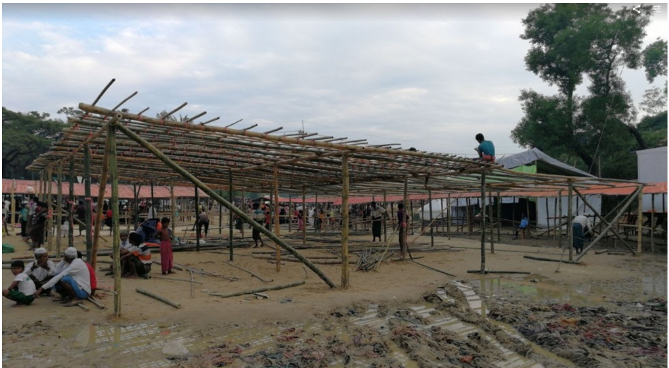
Ongoing shelter construction for new arrivals of Rohingya refugees in Balukhali, Cox's Bazar. @ IOM 2017
