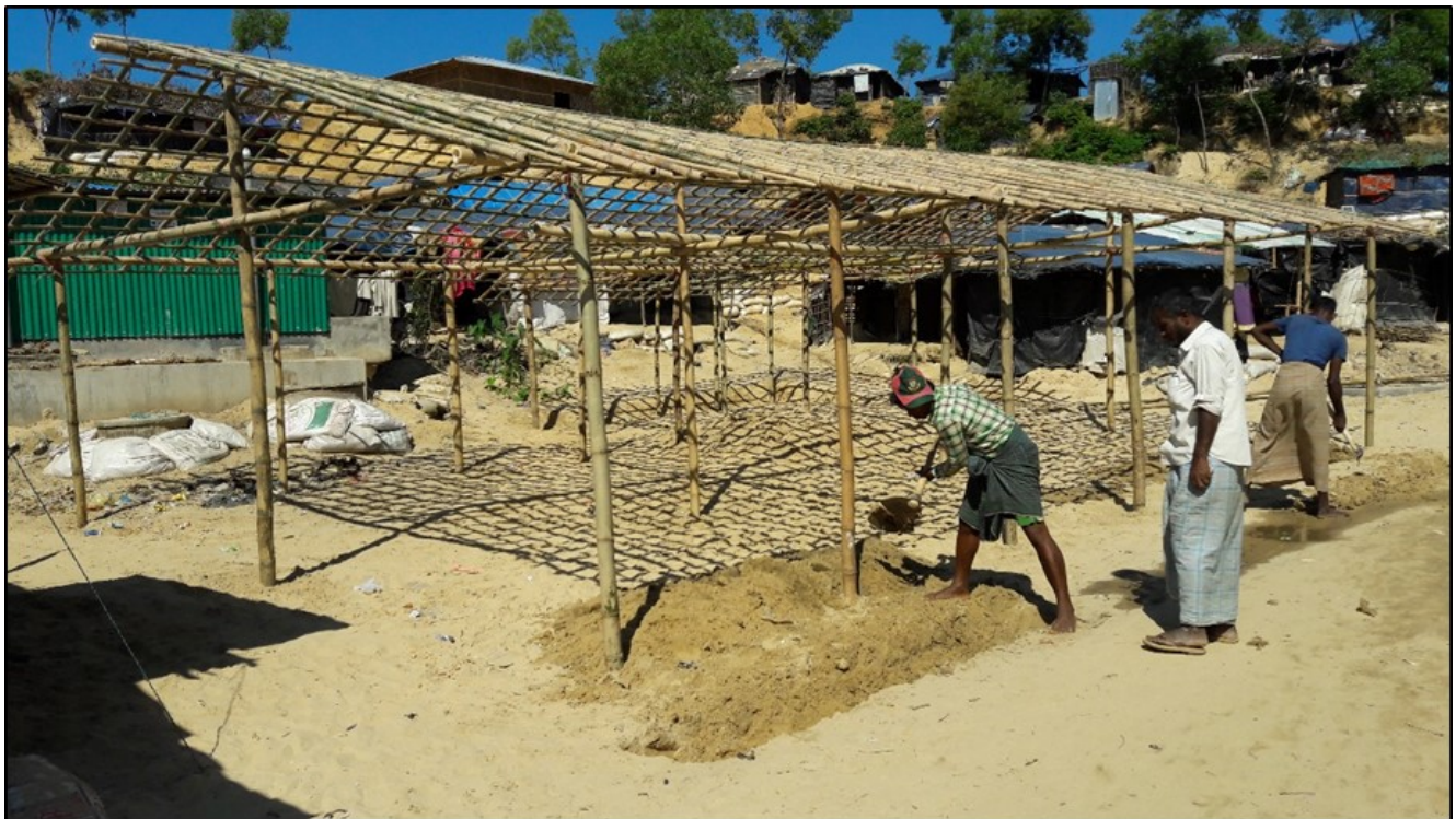
Construction of a temporary health post (tent) in the Kutupalong SS zone that is operational as of 9 Nov. IOM 2017
