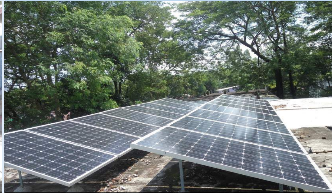
Solar panels are powering health and education facilities on Moheshkhali Island
