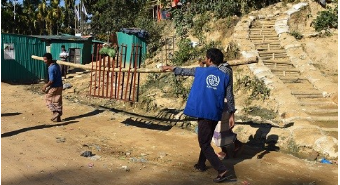
DISTRIBUTION OF IN-KIND MATERIALS FOR SHELTER IMPROVEMENT (TREATED BORAK AND METAL FOOTING) IN CAMP 10. © IOM 2018
