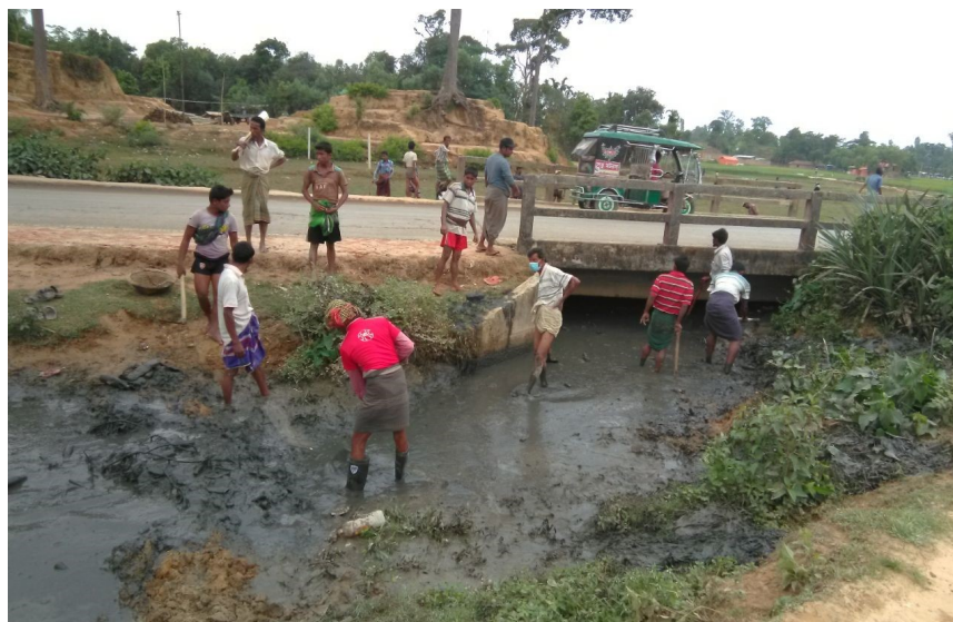
Ongoing clearing of drain at the natural point of discharge (near Cox's Bazar-Teknaf Highway) to minimise water-logging and overflow in adjacent host communities. © IOM 2018
