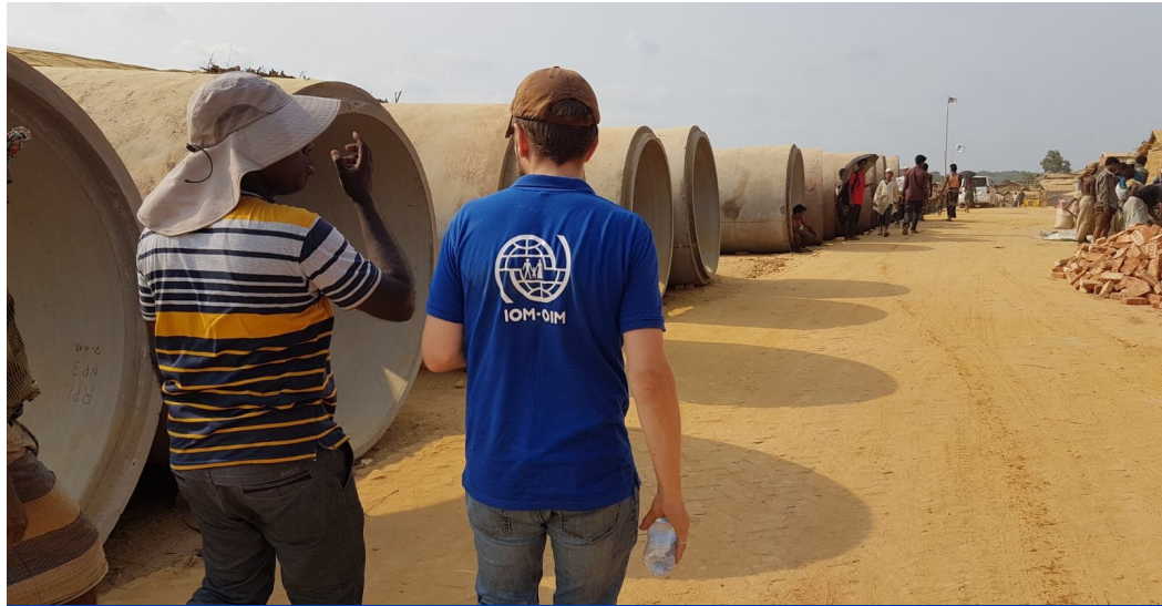
Over 100 culverts have been received and will be installed on Army road in the coming months. © IOM 2018/Fanny Renard
