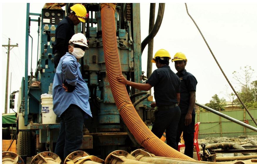
Borehole drilling as part of the joint IOM, JICA, DPHE project in Camp 12.
