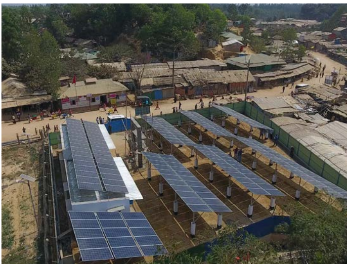
The biggest solar-powered water supply system of the Rohingya crisis, installed in Camp 12, Cox's Bazar, Bangladesh. © IOM 2018
