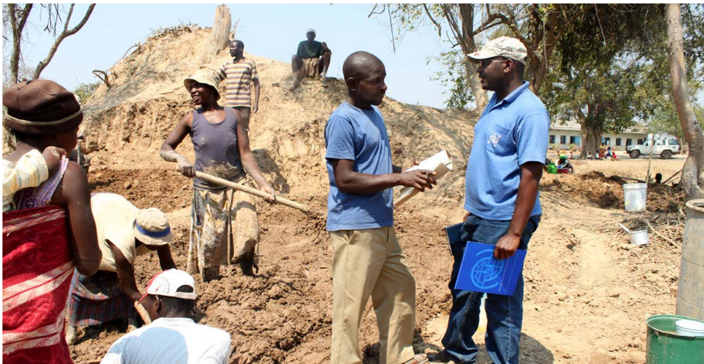
A brick moulding project to facilitate durable solutions for the vulnerable families in Masocha Chisangaurwe Village, Zimbabwe. © IOM 2010 / Judith CHINAMARINGA
