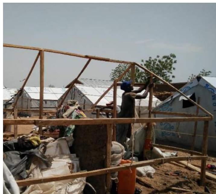
Ongoing reinforcement of old emergency shelters, Umbaza Rockside Camp, Pulka, Borno state, Nigeria © IOM Nigeria 2017
