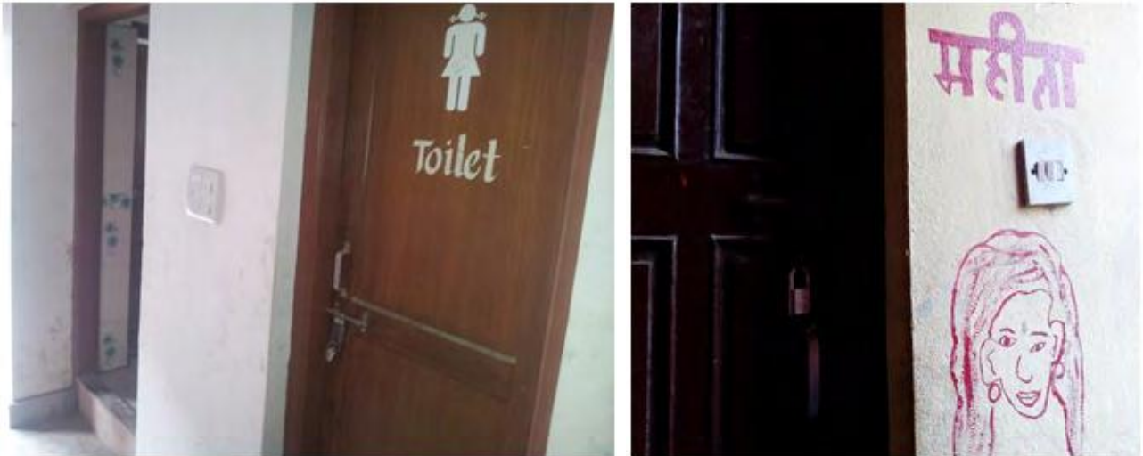
Figure 5: Locked ladies toilets in land revenue offices of Bhaktapur and Lalitpur
