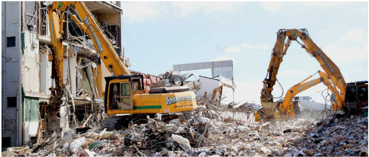
© flickr/Bernard Spragg. NZ – Aftermath of Christchurch earthquake. (CC0 1.0)
