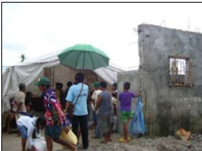
Former health centre of barangay Paya (Giporlos Municipality), a designated evacuation centre entirely damaged by Yolanda Typhoon (March 2014).
